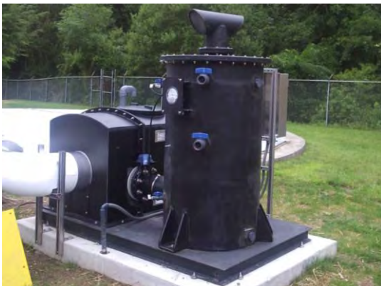
Lo-Flow Unit installed as part of a skid system
